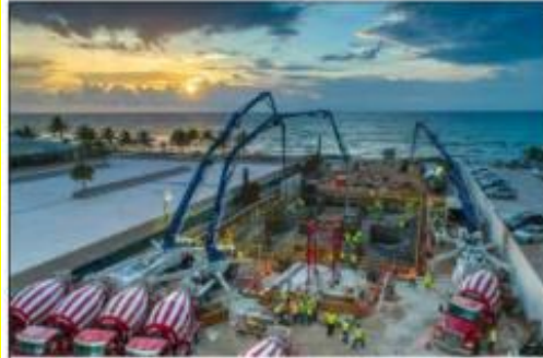
2000 Ocean Foundation poured Suffolk Construction had an epic pour of 2,483 cubic yards of concrete for the foundation of KAR Properties' 2000 Ocean in Hallandale Beach. Amy Ballion of Fortune Development Sales Group was appointed as the sales director for the 38-story beachfront condominium property.
